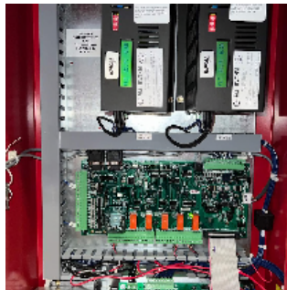
Diesel Engine Controller
