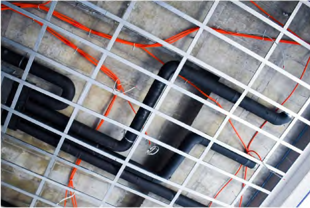
Ducts, Plenums, and Other Air-Handling Spaces
