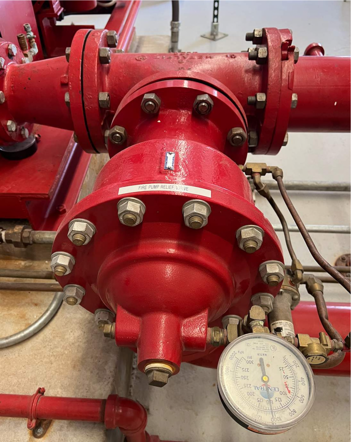
A shutoff valve is not permitted in the relief valve supply or discharge piping.
