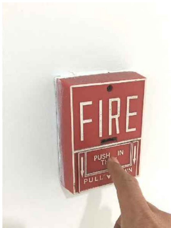
Manual Fire Alarm Boxes
